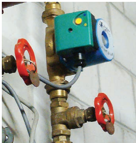
ONE OF THE ULTRAFLOW CIRCULATION PUMPS
